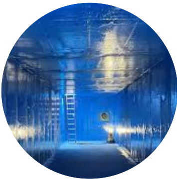
Process water containment
